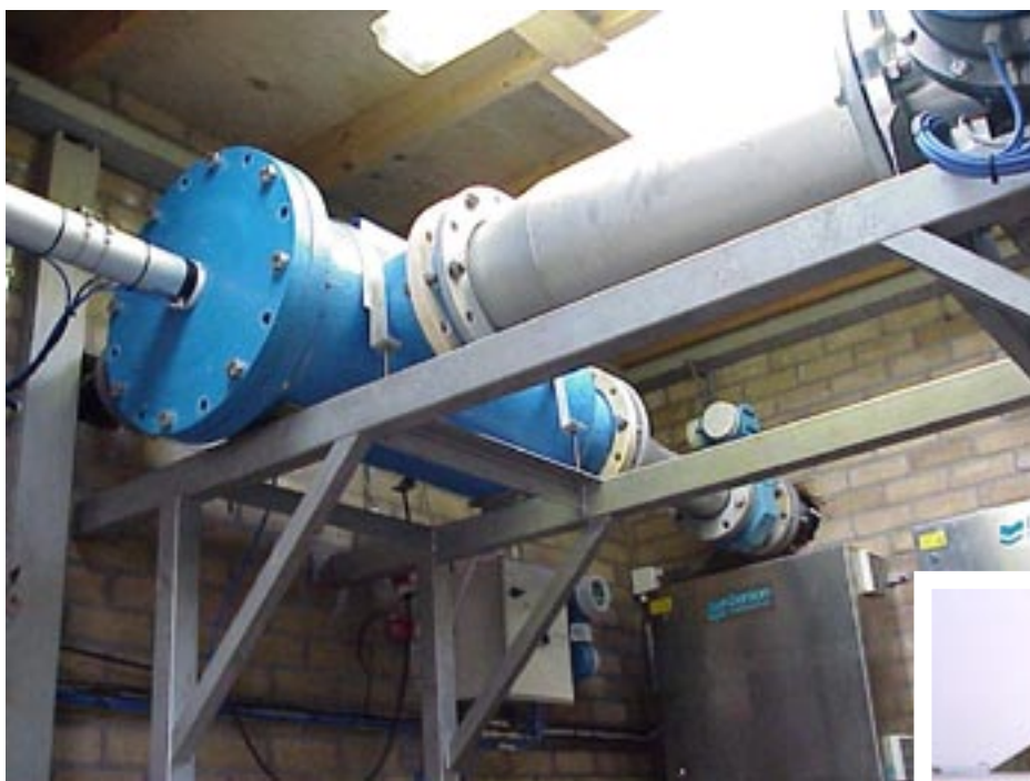
Bernoulli Filters as pre-filters before UV disinfection units for sea water intake in mussel production plant.
